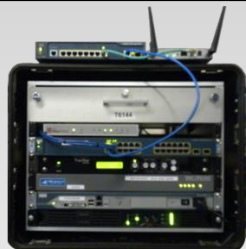
Dismountable Network Rack
